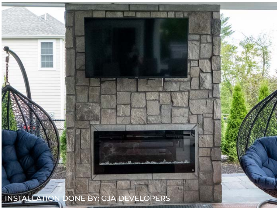
INSTALLATION DONE BY: GJA DEVELOPERS
